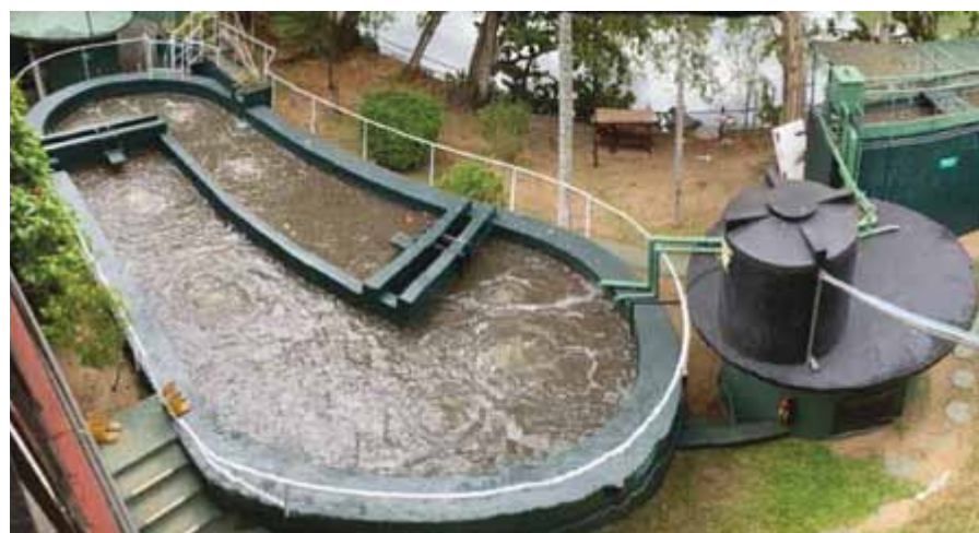
Water treatment plant 'Cinnamon Citadel Kandy'.
