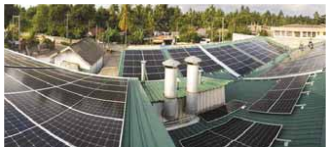
Solar panels installed at the KFP factory.
