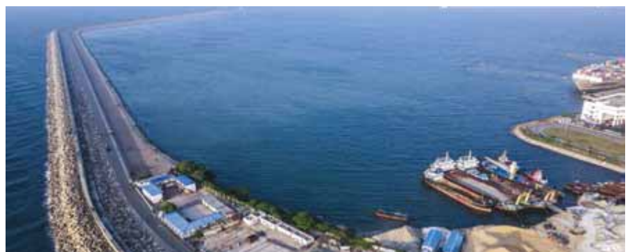
The WCT-1 site was handed over in February 2022 for the commencement of construction.
