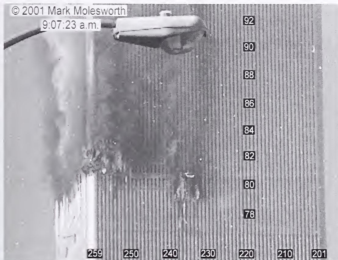
Figure 9-8. This image captured from a video shows the north face of WTC 2 at 9:07:23 a.m. Column and floor numbers have been added.
