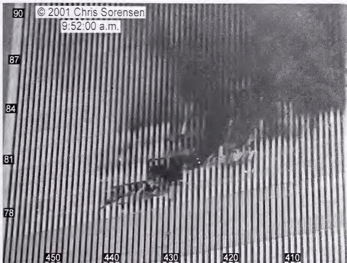
Figure 9-68. This view of the south face of WTC 2 was taken from a video recorded at 9:52:00 a.m. The intensity levels have been adjusted, and column and floor numbers have been added.
