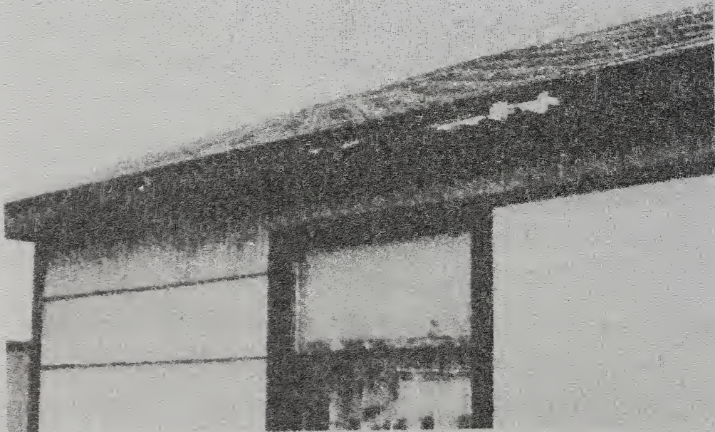
Figure 13 Paint failure due to drying operation. Ventilation of attic space will assist in reducing failures of this type.
