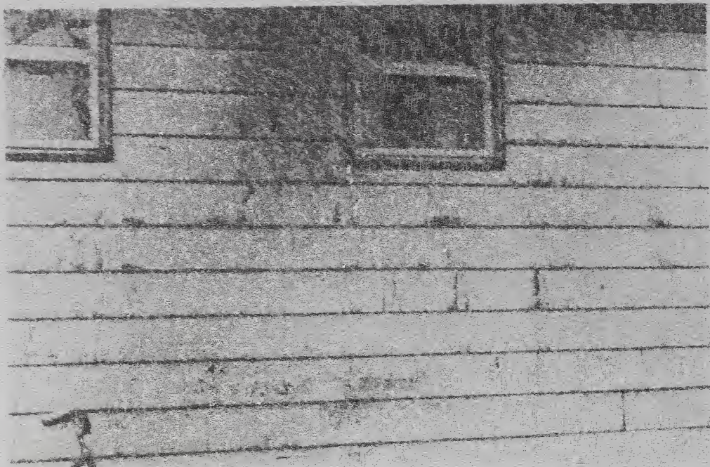
Figure 8 Staining of exterior siding due to forced drying procedure.
