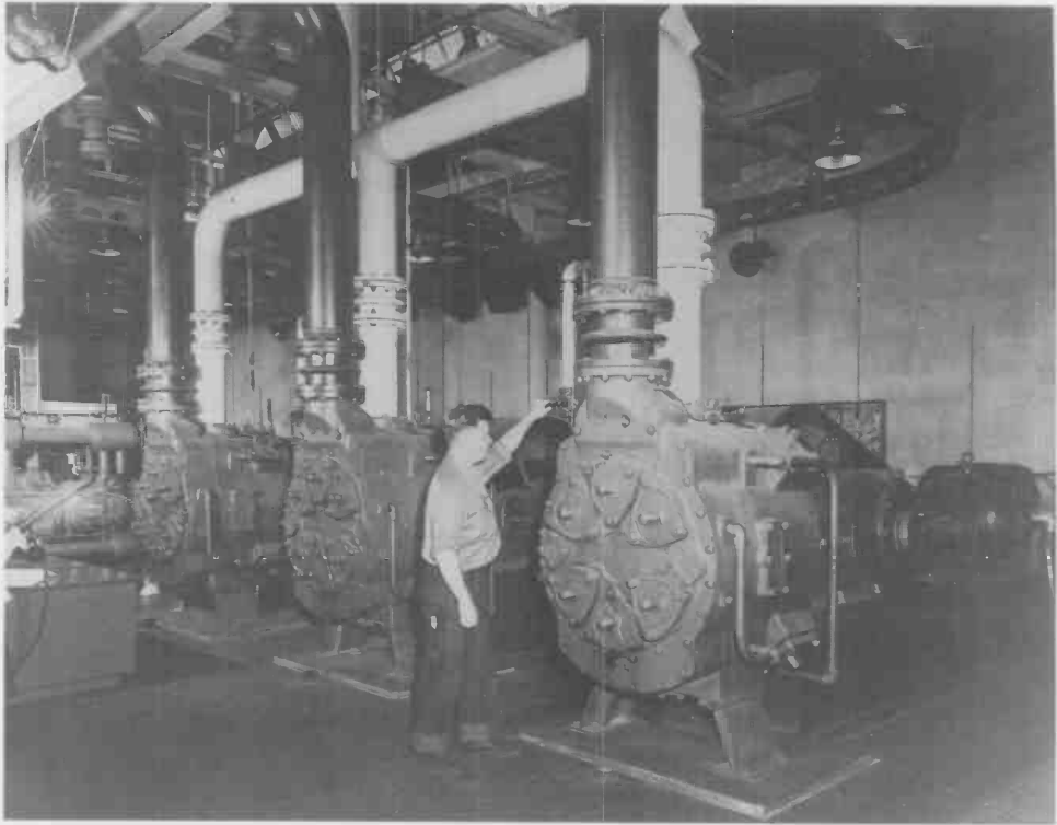
Large reciprocating vacuum pumps in the hydrogen liquefaction plant of the NBS-AEC Cryogenic Engineering Laboratory. These pumps were used to reduce the boiling pressure—and hence the temperature—within the liquid-nitrogen precooler. Dean B. Berkly is shown opening the vacuum breaker on the first of the three vacuum pumps.
