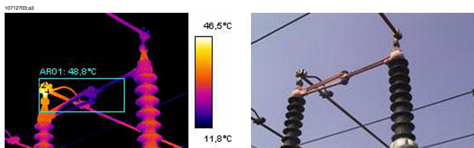
Figure 29.1 An infrared and a visual image of a power line isolator
