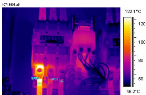
Figure 29.9 An infrared image of indoor electrical equipment (2).
