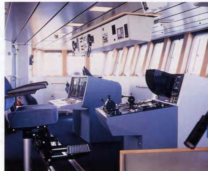
View from the Bridge with Consoles to the left containing workstations for the Ship Control and Supervisory System and to the right for controlling the Propulsion and Maneuvring System
