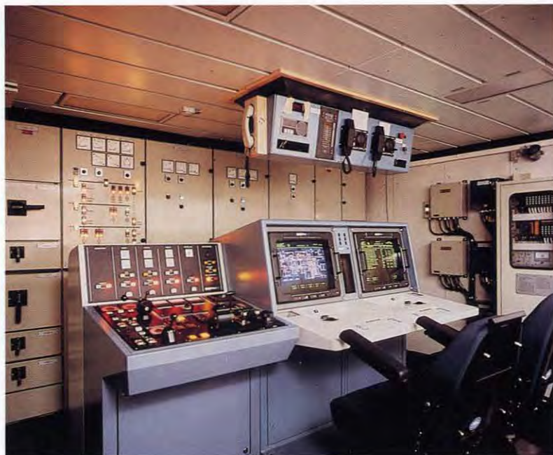
Consoles for the Machinery and Propulsion Plant Control and Alarm System
