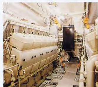
STELLA ® computer outstation in the engine room
